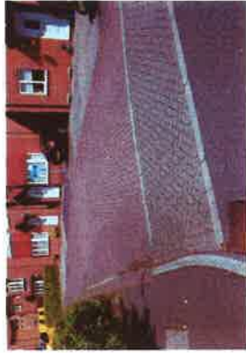
Raised table at the entrance to a minor route with block paved shared vehicular / pedestrian space.
