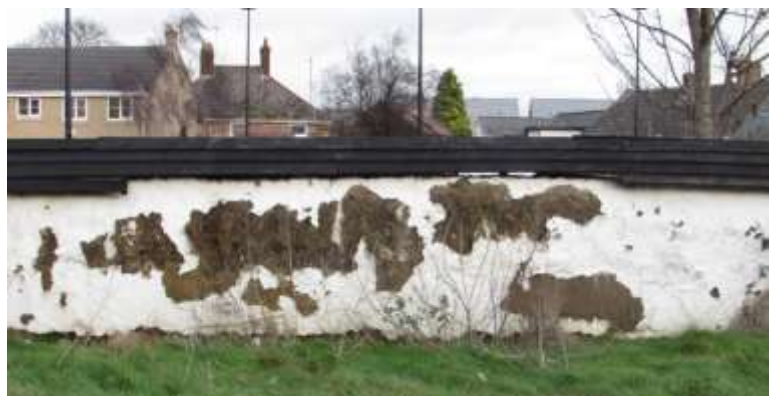
Scaffolding and deteriorating mud walls
