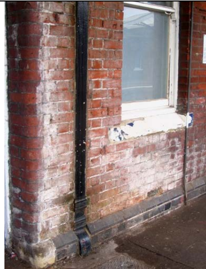
Brickwork condition, down side buildings
