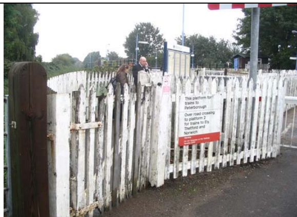
Access to down platform – paling fence in poor condition.
