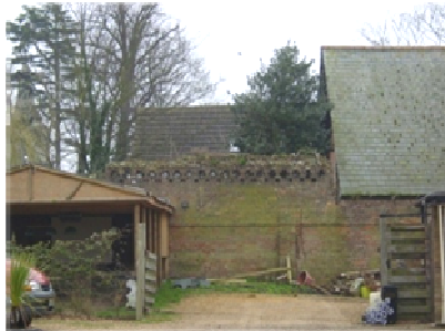
Sensitive repairs are needed to the stretch of wall between The George Public House and Church Rooms.
