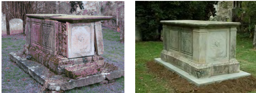
Above: An early 19 th C chest tomb in Doddington churchyard (before and after restoration with a Fenland District council grant).
