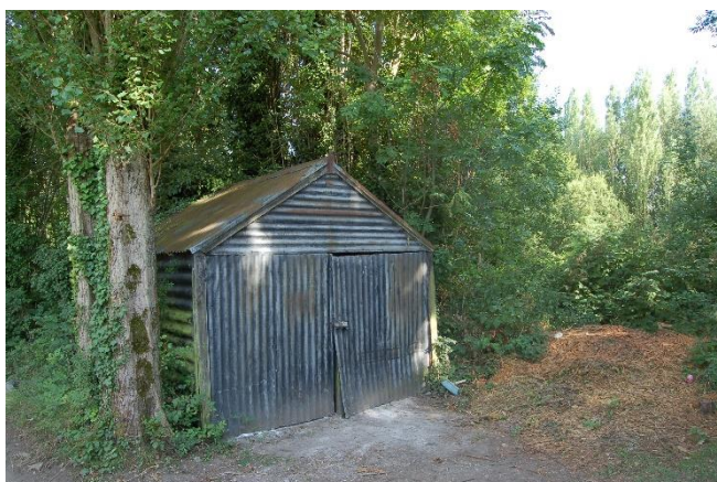
Photograph 14 Building 3 which represents the typical type of outbuilding present within the northern half of the site
